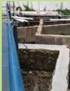
Instalasi Sediment Pond pada Proyek Sequis Tower / Sediment Pond Installation at Sequis Tower Project
