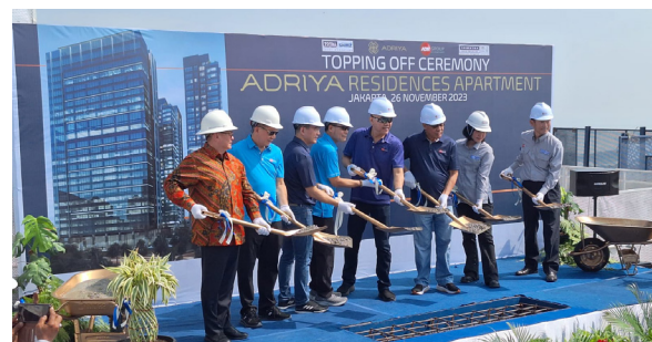
PROSESI PENUTUPAN ATAP (TOPPING OFF) PROYEK PIK ADR A TOPPING OFF CEREMONY AT PIK ADR PROJECT
